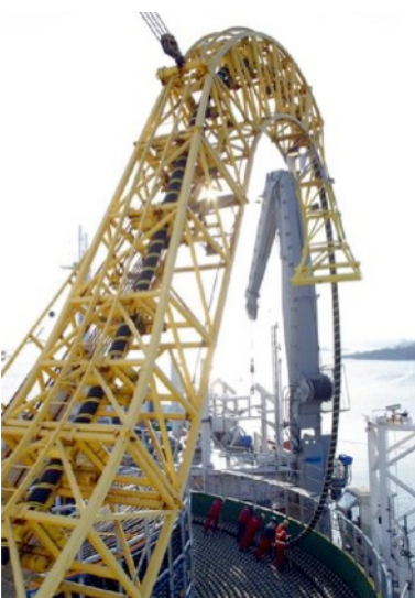
An undersea HVDC cable laid by this ship now enables Norway and the Netherlands to share wind and hydropower. With only a small part of its budget the EU could accelerate the construction of links like this across the region.
