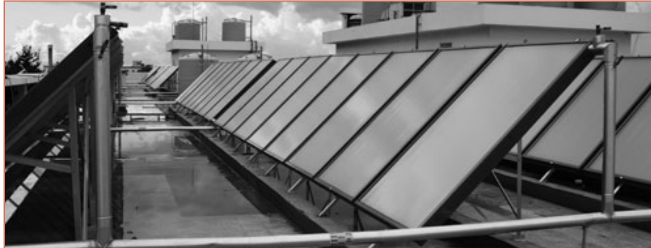
Solar roofs at Tripoli Public Hospital Image provided by: Rola Khazen, Lebanon
